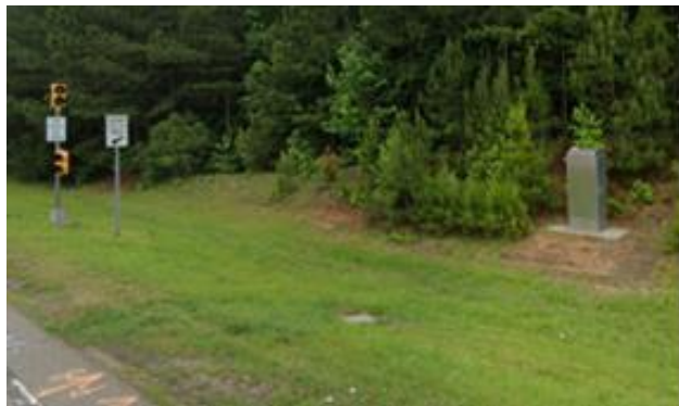
Figure 10: Example of Typical Controller Cabinet Placement
