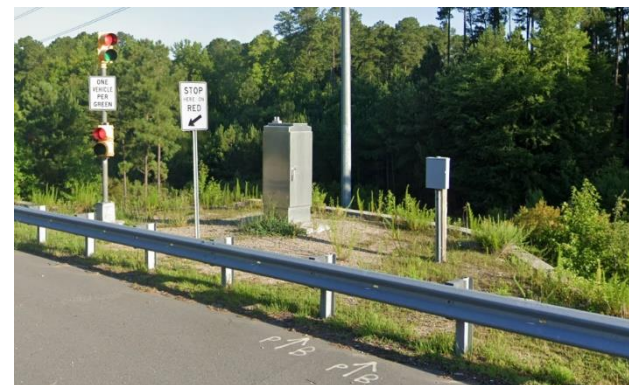
Figure 11: Example of Controller Cabinet Placement Requiring Grading and Guardrail
